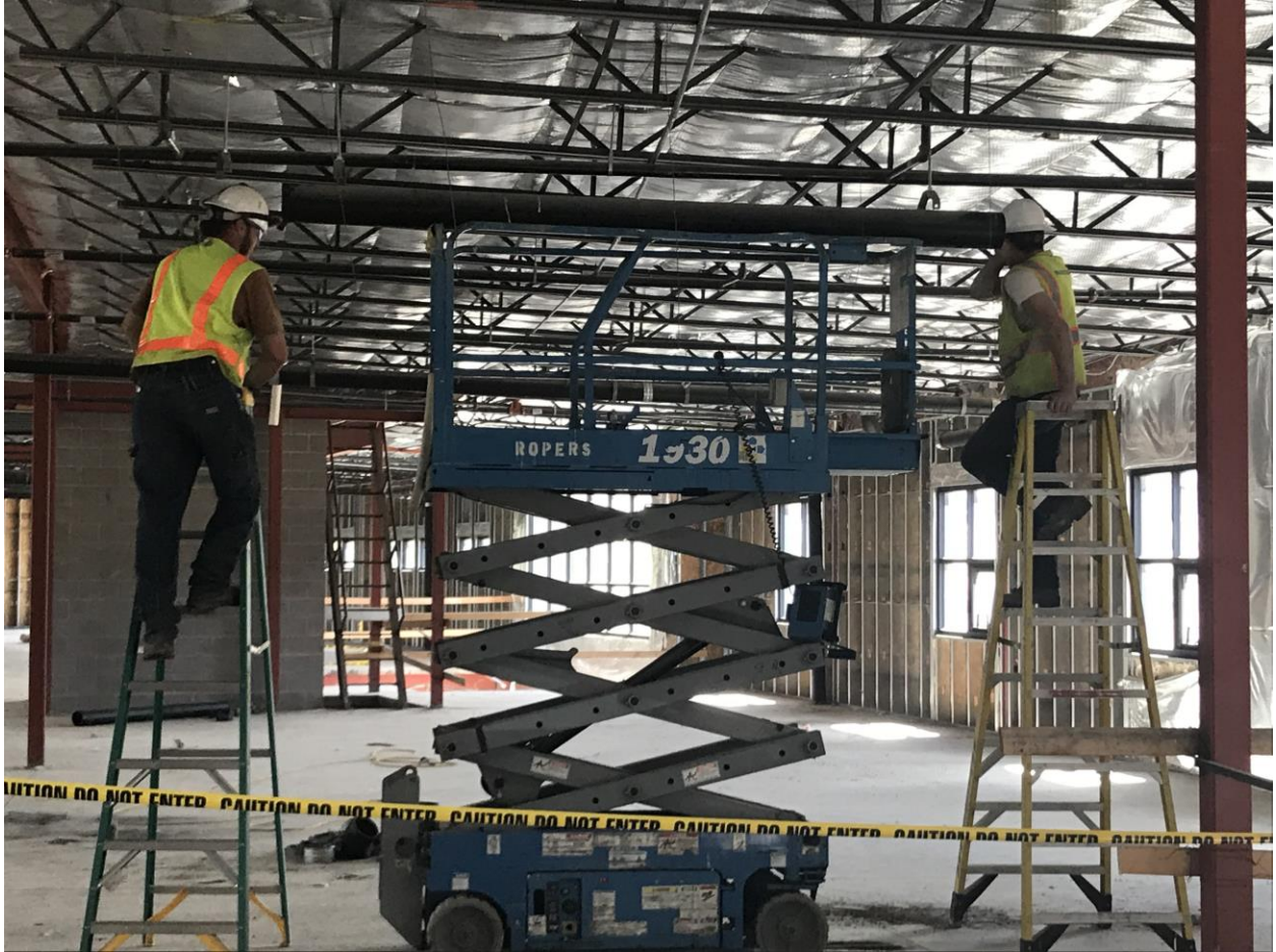
Caption: Construction crews from HB Construction are working to complete county offices in the Mora County Complex.
